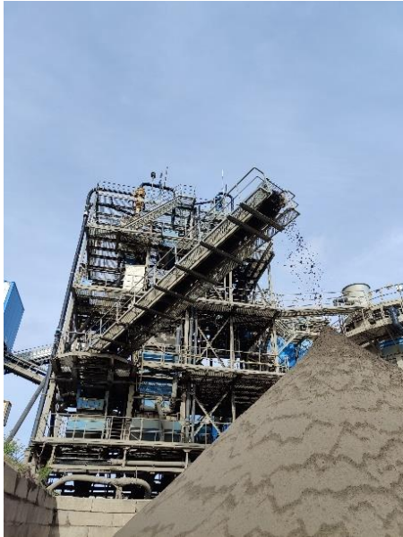
Washing installation BIOTERRA NV
